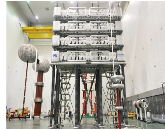
\pm 535 kV/3000MW converter tower
